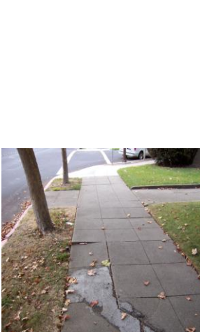
Roots raising sidewalk
