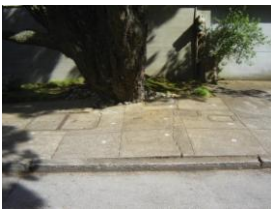
Before: Damaged sidewalk by Monterey Pine
