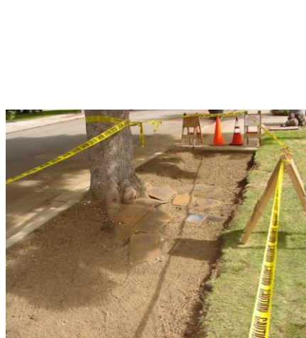
Sunnyvale, CA steel plates over roots
