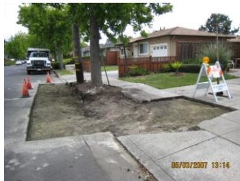
Large roots under sidewalk and driveway
