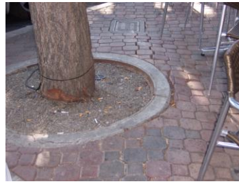
Concrete ring raised by roots Trunk is so large the grate was replaced with DG
